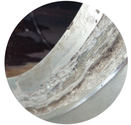
Corrosion caused by use of conventional graphite gasket
